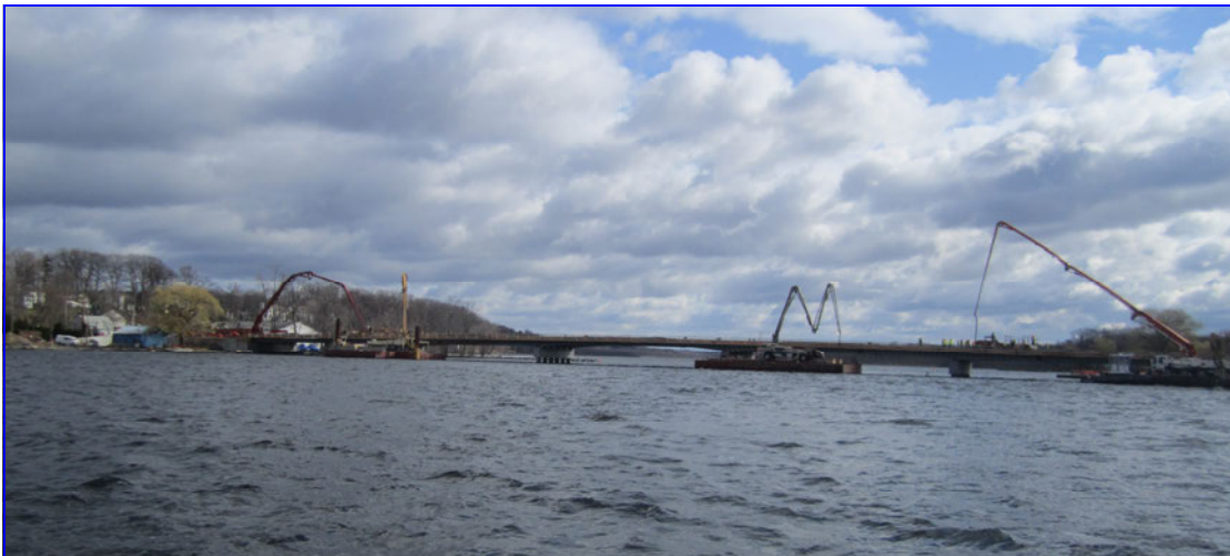
Concrete pump trucks deliver concrete to the new bridge during deck pour #2.
