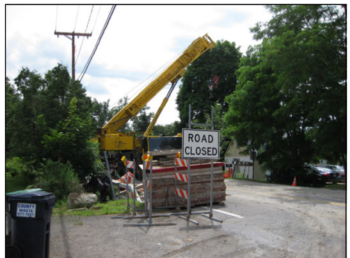
Work is progressing at the culvert site on Route 9P and Brown Road.
